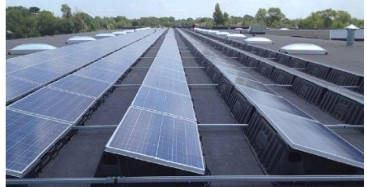
Ballasted Flat Roof Solar Power Systems
